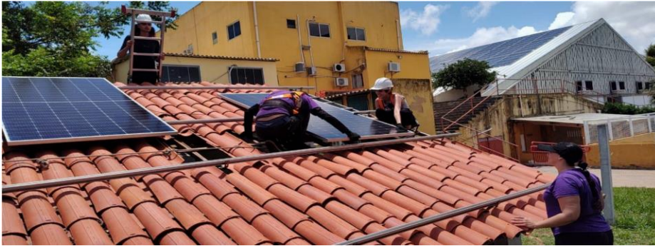
Figure 4 - System assembly photovoltaic on the roof didactic.
