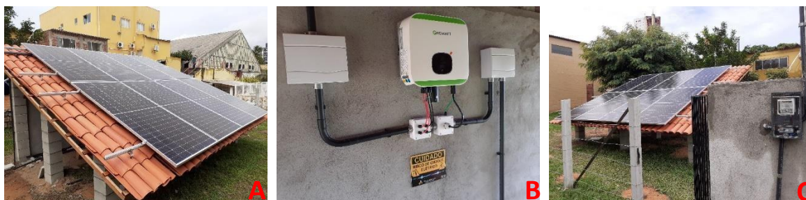
Figure 3- Roof didactic installed at IFRN III. WORK SAFETY AND ESSENTIAL STANDARDS
